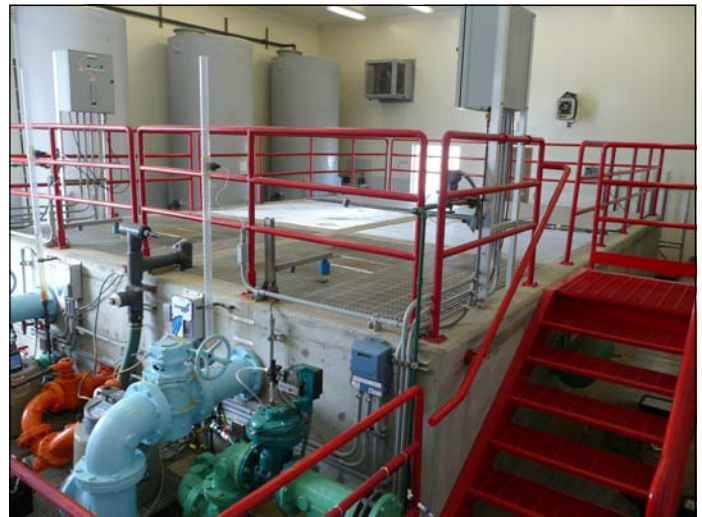
Blue PRO ® 1.5 MGD Installation
